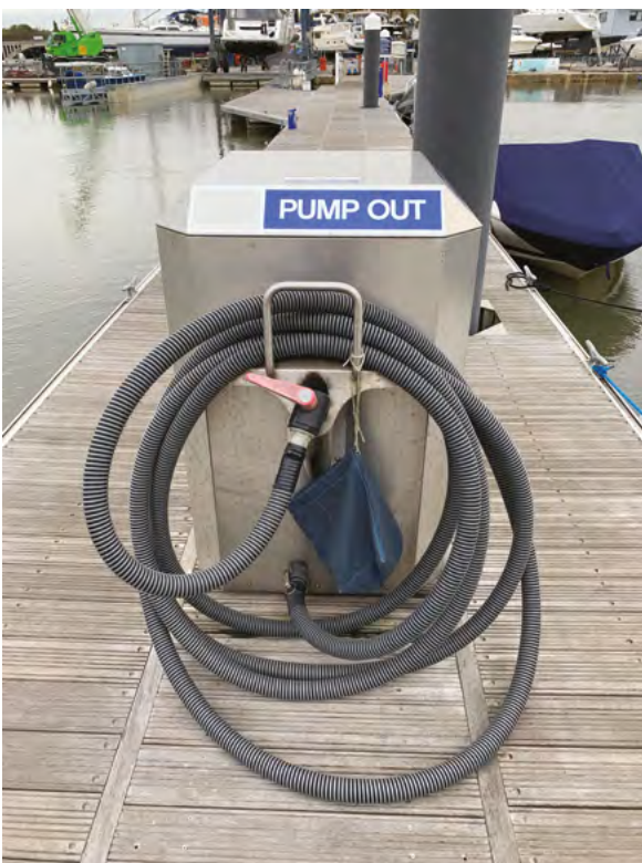
C. Pump out station
