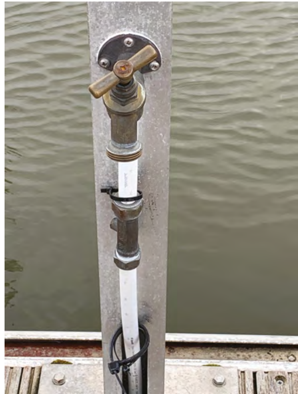
B. In-line Double Check Valve (DCV) (insulation removed)
